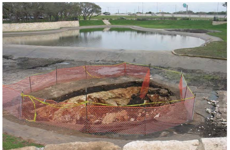
Sinkholes and other karst problems are more likely to occur without good advance site characterization. Site in south Austin, Texas. Courtesy of the Brians (BSEACD).
