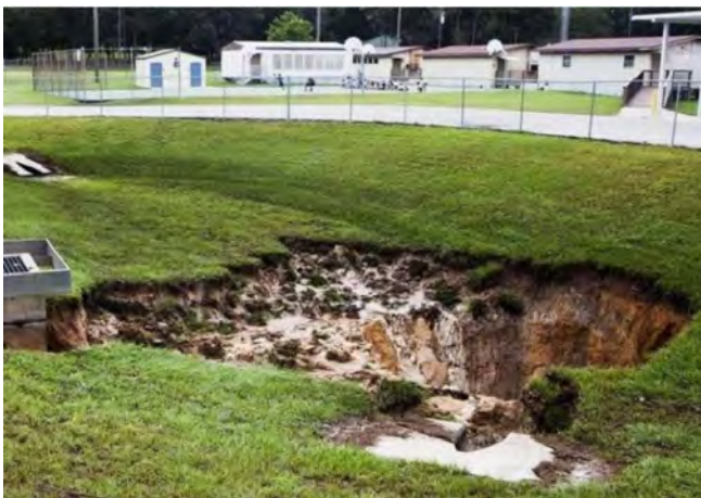
Improper stormwater designs can lead to future problems.
